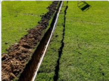
Structured cabling Data cabling run properly for cameras, Wi-Fi and networks, by a registered open cabler. See structured cabling
